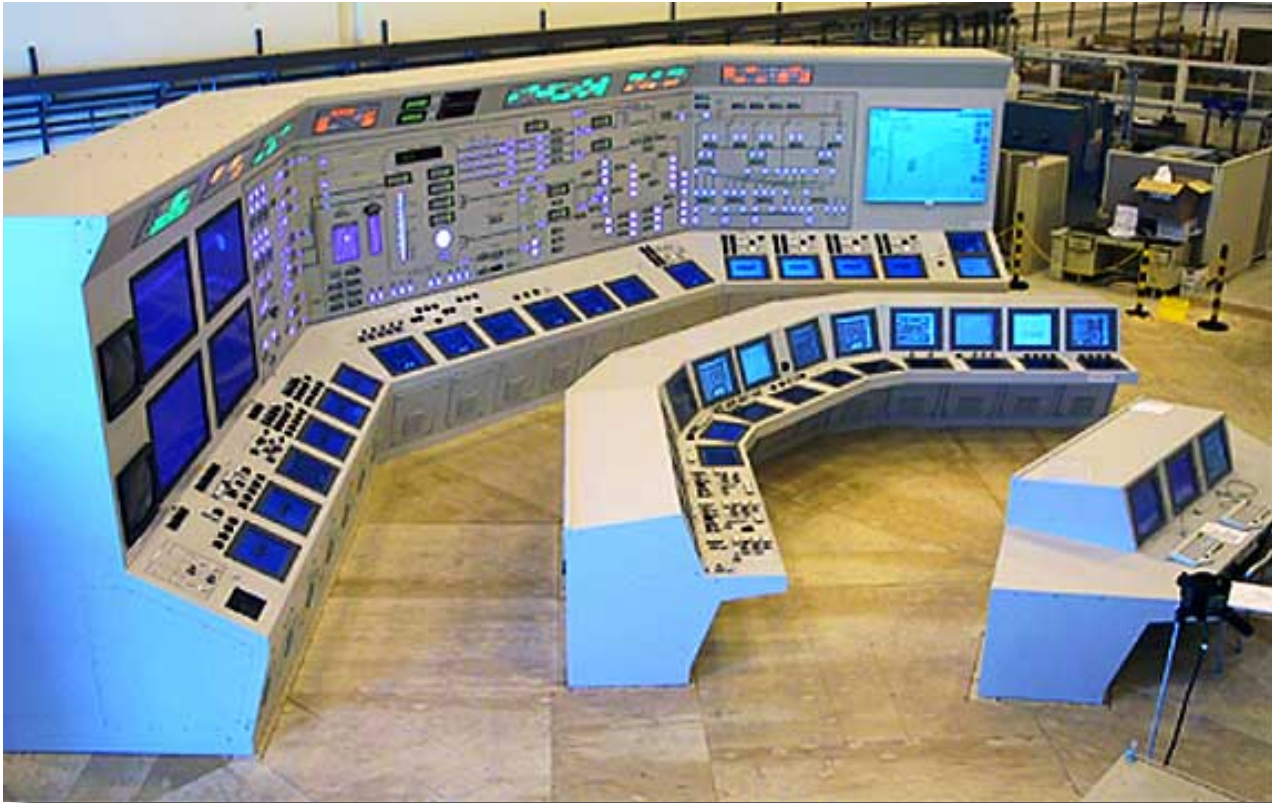
Figure 2-5. ABWR (Lungmen) Main Control Room Panels
